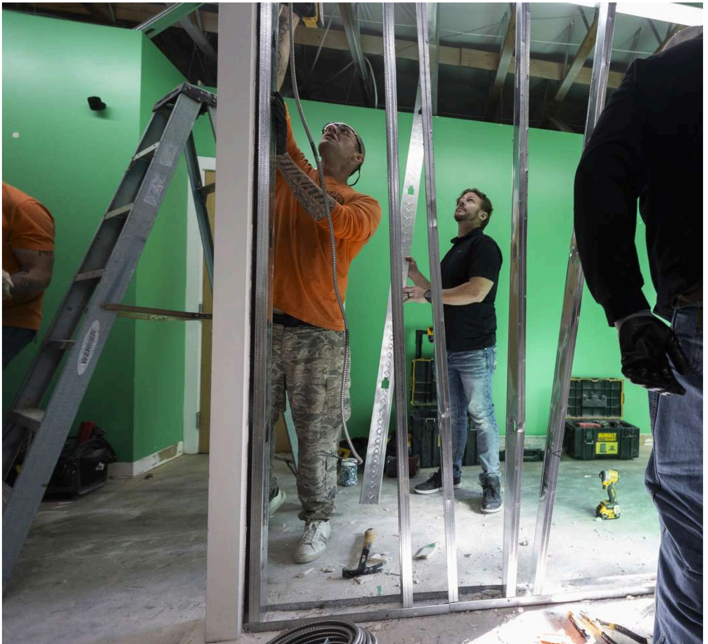
Students from the Other Side Academy work on building a expansion for Habitat for Humanity's office in Salt Lake City on Monday. (Photo: Brice Tucker, Deseret News)
